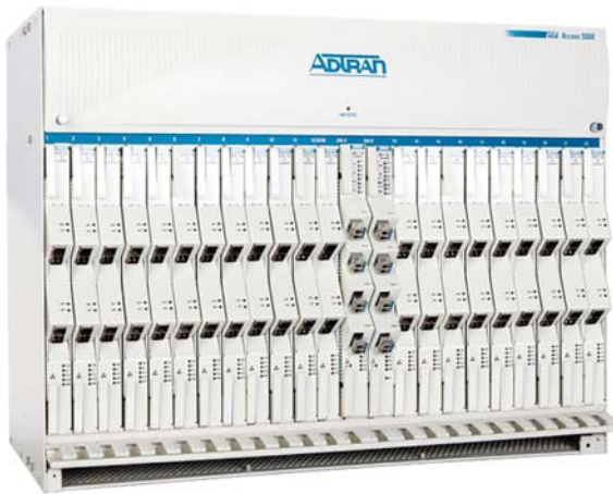
Figure 4-11 An Optical Line Terminal with ports on cards where fiber is terminated in central offices. (Photo courtesy of Adtran Inc.)
